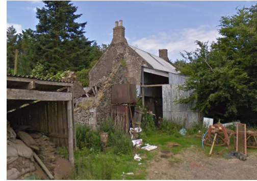
Ruined Farm Houses Stone Walls Sinusoidal metal Roof cladding
